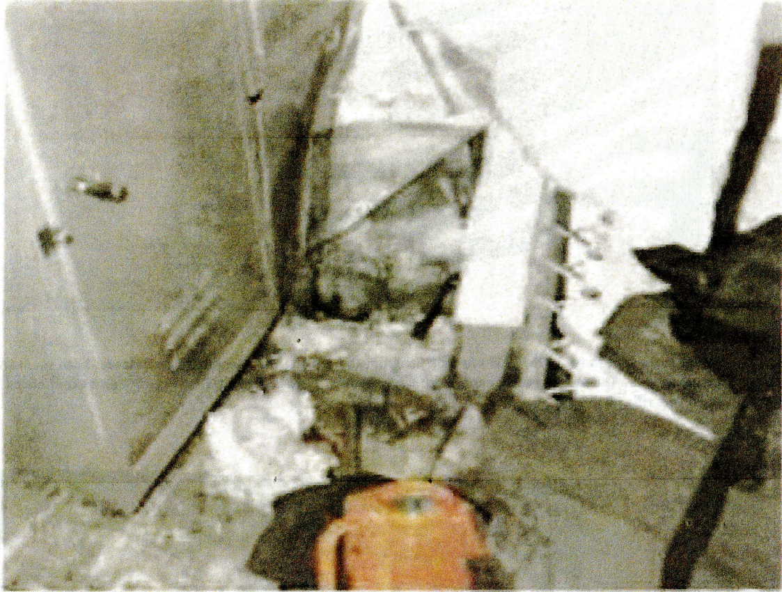
Figure 7: More damage control
